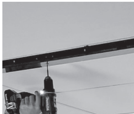
IV.13. Pre-drill \frac{1}{2} holes on the bottom side of top horizontal profile. Be careful not drill through the top side of the profile.
